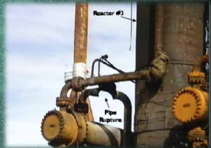
Element 15 Case Study: Tosco Avon Refinery, Martinez, CA. January 1997
