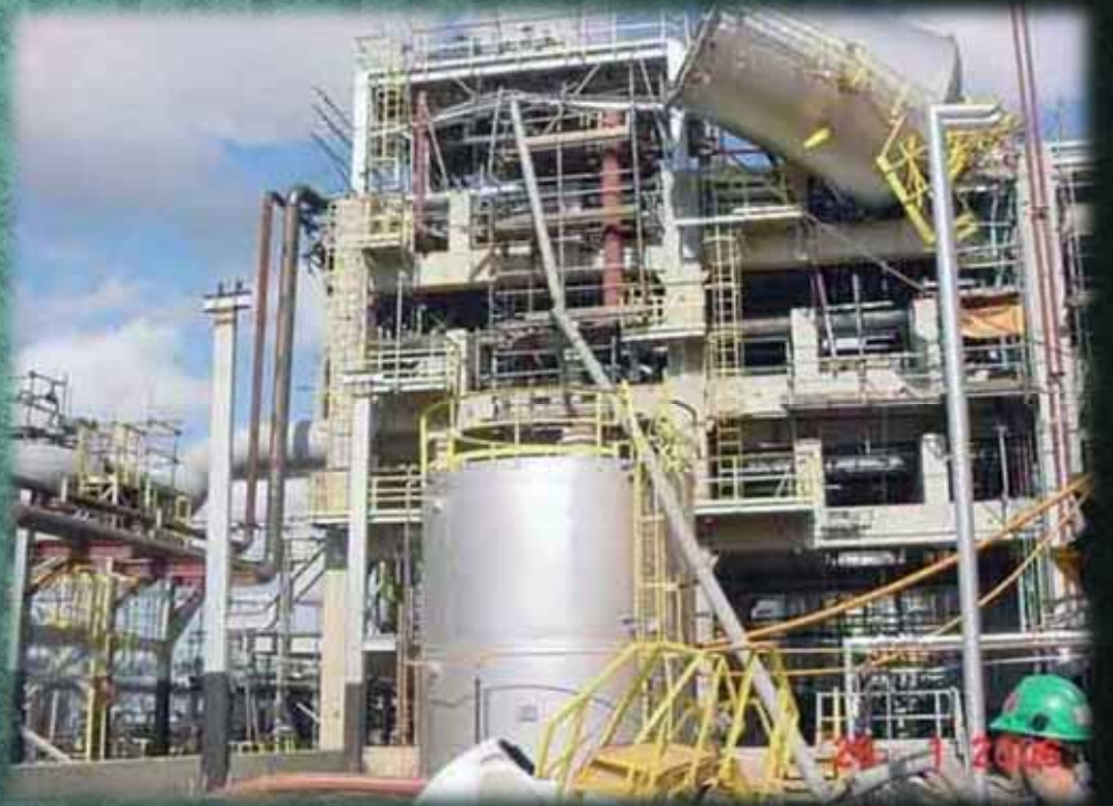
Element 14 Case Study: Pneumatic Testing Accident, Brazil January 26, 2006
